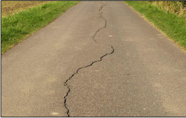
Photograph showing Longitudinal Cracking.
