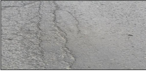
Photograph showing Centre Cracking
