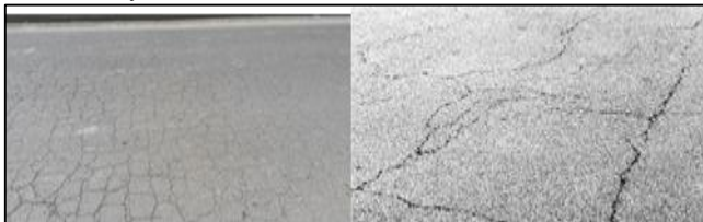
Photograph showing Block Cracking
