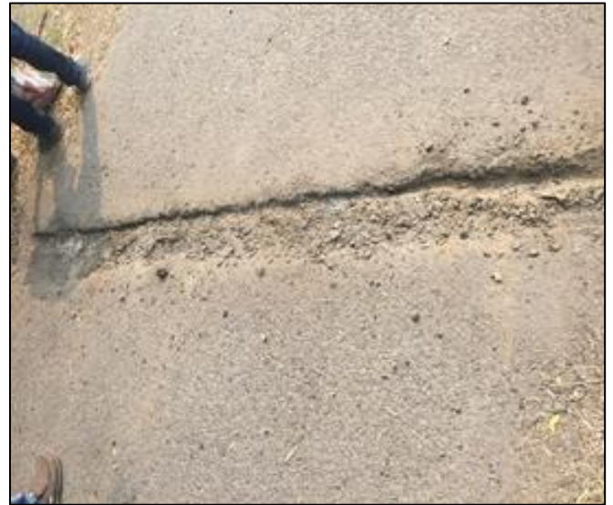
Fig. 13: Pothole in NTPC badarpur
