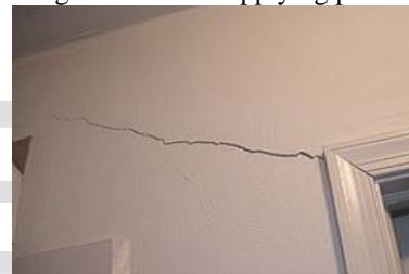
Fig. 6: Shows vertical crack & spoiling of concrete in RCC Beams
