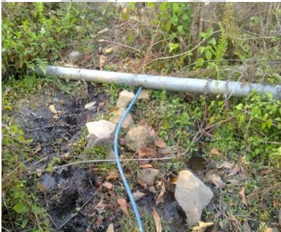
Fig. 18: Illegal stealing of water from the PHED pipes
