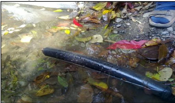
Fig. 7: A plastic pipe with holes pierced on the sides for intake from the river
