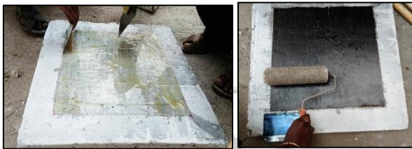
Fig. 4: Application of the resin(a) and fabric is placed and rolled with roller(b).
