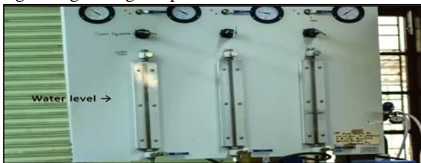
Fig. 5: Water Level Indicator for Water Reservoir
