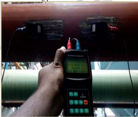
Fig. 2: Takes Reading From Ultrasonic Flow Meter
