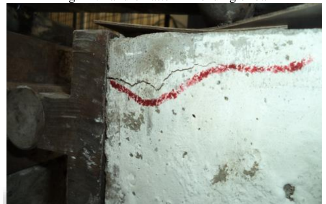
Fig. 15: Crack Pattern near hing
