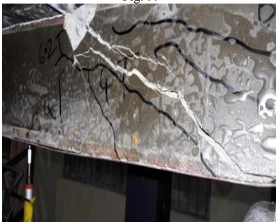
Fig. 10: Typical failure of RC strengthened beam with continuous steel sheet (1.5mm) at bottom and Side faces
