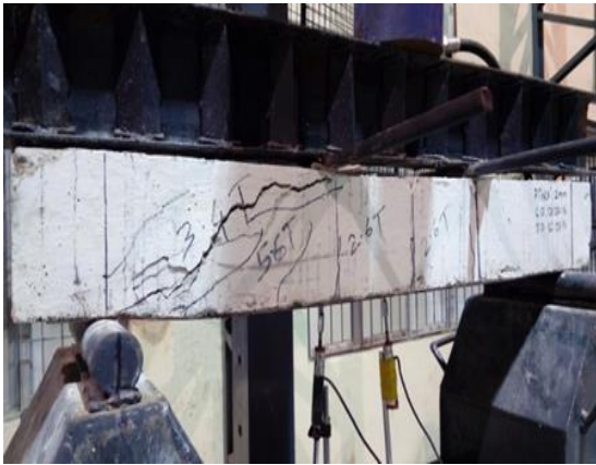
Fig. 8: Typical failure of RC strengthened beam with continuous steel sheet (2 mm) at bottom
