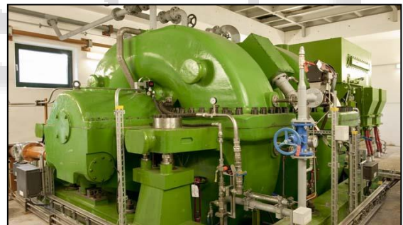
Fig. 2: Gas Expansion Turbine
