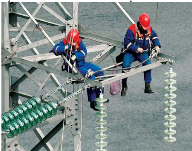
Fig. 7: Safety To Personnel
