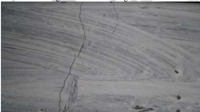
Fig. 6: Crack in Tension Zone Propagates in Upward Direction
