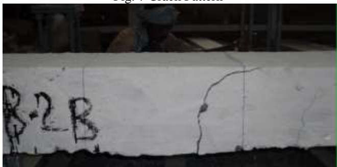
Fig. 8: Failure of 2nd group of beam at Ultimate Load
