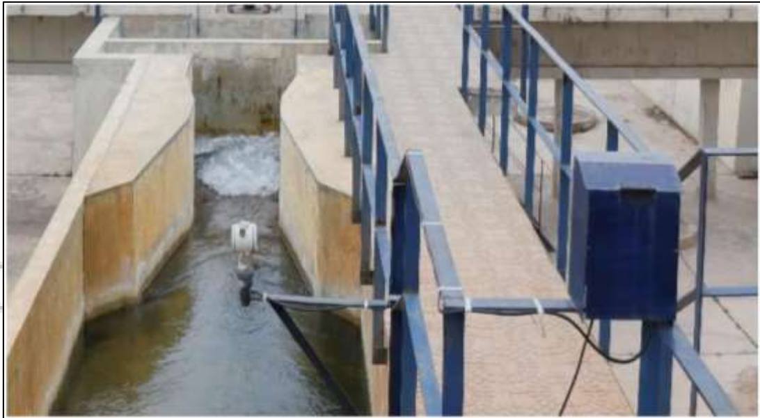
Fig. 2: Ultrasonic Flow Indicator over Parshall Flume
