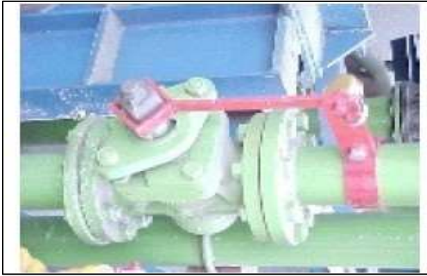
Fig. 3: Example of Valve LOCKOUT
