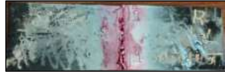
Fig. 3.4: defects on root weld
