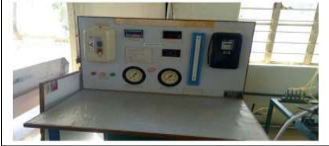
Fig. 1: Compressor Indicator board
