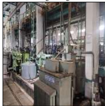
Fig. 2.2: Copper Plating Plant
