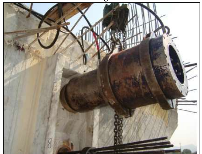
Hydraulic Jack for Post Tensioning
