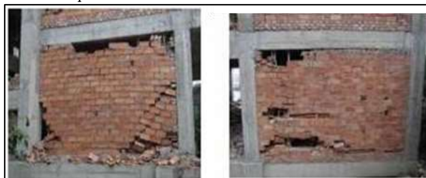
Fig. 1: a) Infill Compression and Shear damages b) Infill compression and Minor frame and minor frame Damages
