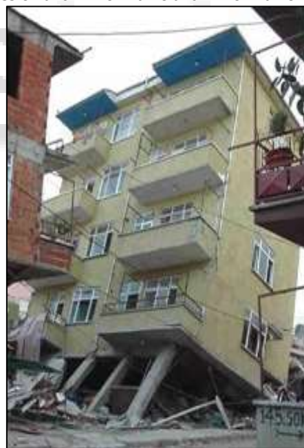
Fig. 2: Partial collapse of RC frame building with masonry infill walls in Yingxiu during Wenchuan earthquake.
