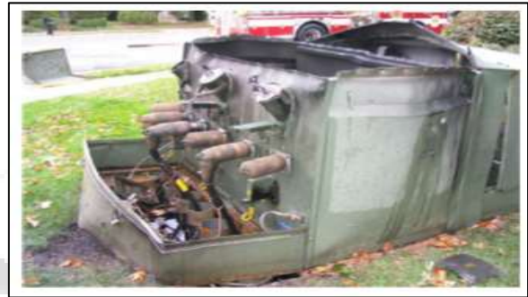
Fig. 2: the mineral oil leakage after a 19kv transformer explosion.
