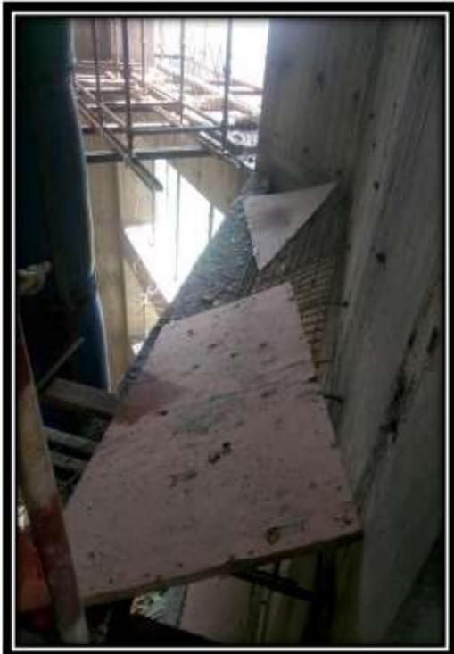
Fig. 3: Falling hazard which has been barricaded
