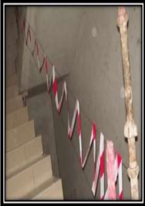
Fig. 4: Falling hazard on the stair edges which has been barricaded
