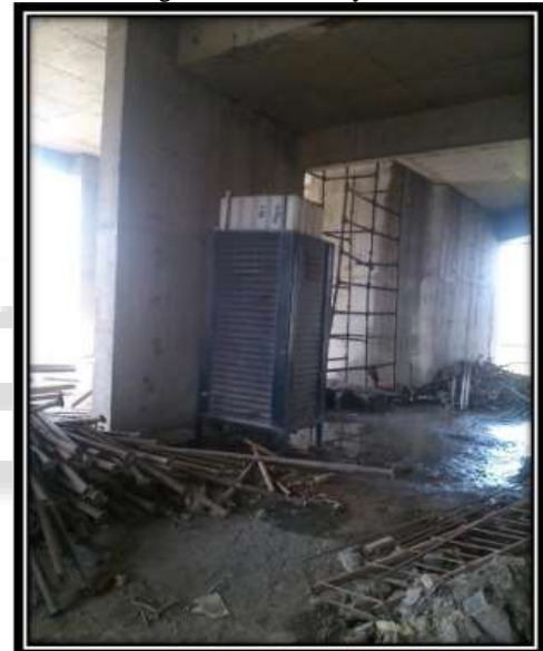
Fig. 10: On-site Sanitary Conditions
