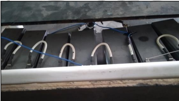
Fig. 5: Lead Acid Battery
