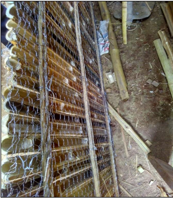
Fig. 1: Wire Mesh Layer on the Inner Part of Wall Panel before Plastering
