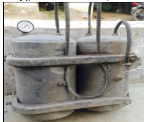
Fig. 2.3: Compressed Air Tanks
