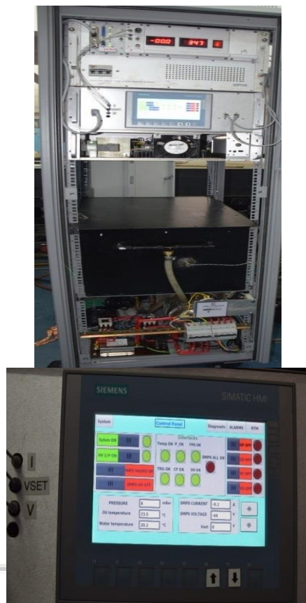
Fig. 7: (A)controller unit in 39U rack and (B) zoom view of HMI screen.
