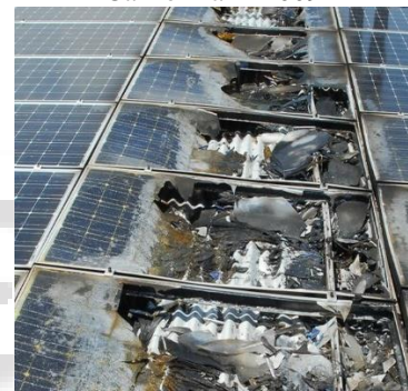
Fig. 1(b): fault occurred in 1 MW PV power plant in Mount Holly, North Carolina, in 2011
