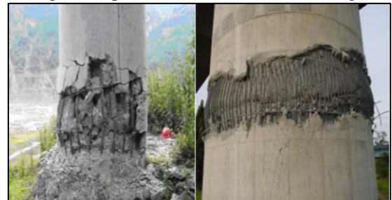
Fig. 3: Damages in Pier
