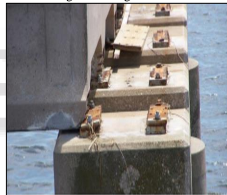
Fig. 4: Damages in Bearings
