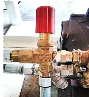
Fig. 13 Pressure relief valve Pressure switch
