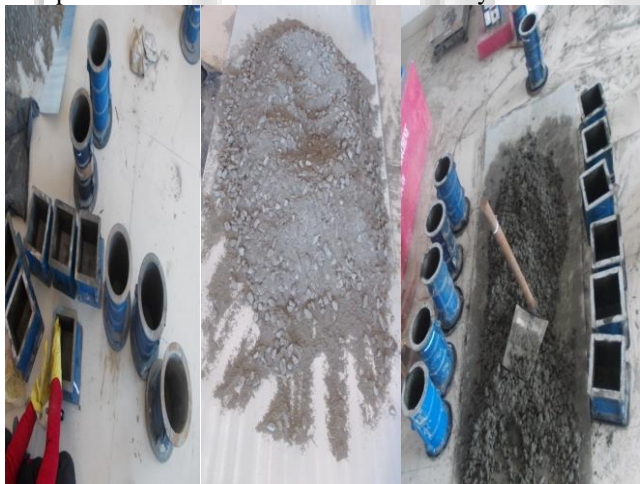
(A) Oiling of Cubes & Cylinder (B) Dry mixing (C) Filling of Moulds Fig. 1: Casting
