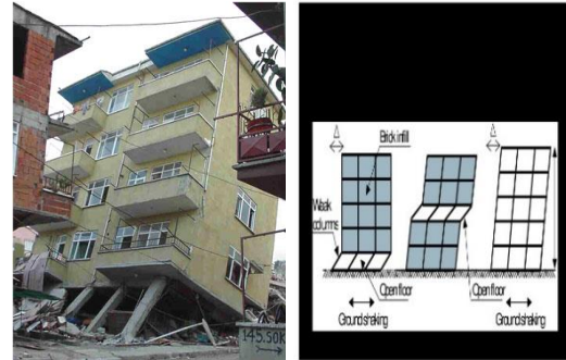
Fig. 3: (C) Ground Soft Storey Failure Fig 3(D) Soft Storey Failure Pattern
