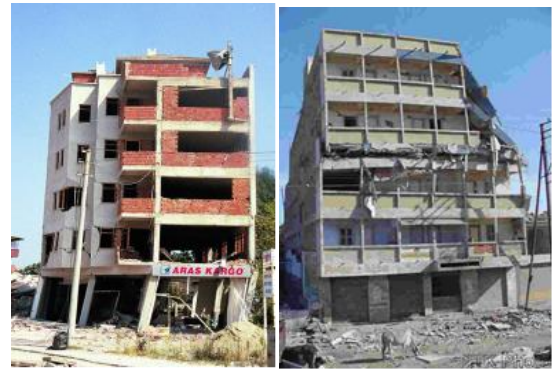
Fig. 3: (a) Ground soft storey failure, Fig 3(b) Intermediate soft storey failure
