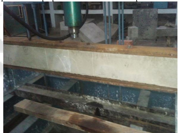
Fig. 5: Beam two is retrofitted with double plates top and double plate bottom of the beam
