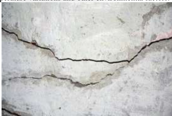
Fig. 1: Cracks formed in structure
