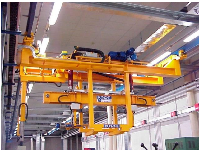
Fig. 1: Example: Overhead Crane used in Material Handling
