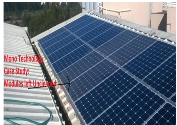
Fig. 6: Make: Shan Solar (255Wp per Module)
