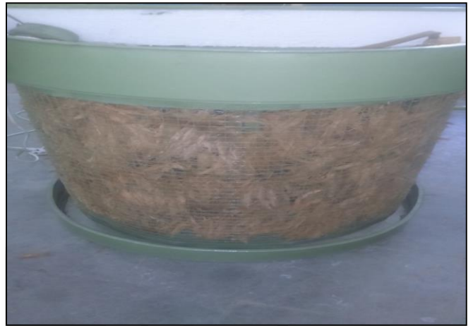
Fig. 10: Coconut pad material in evaporative cooler
