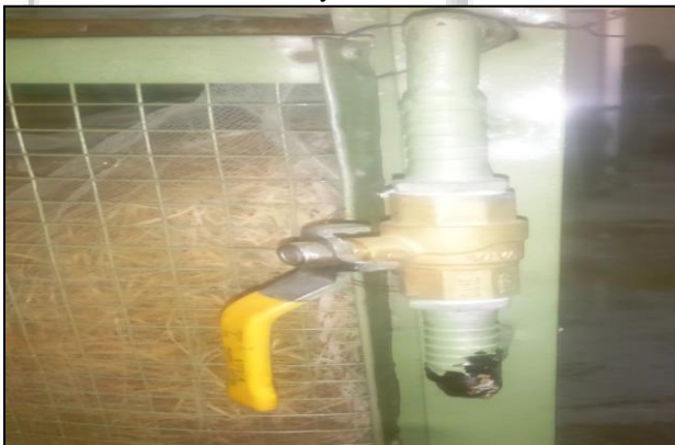
Fig. 4: Flow control valve
