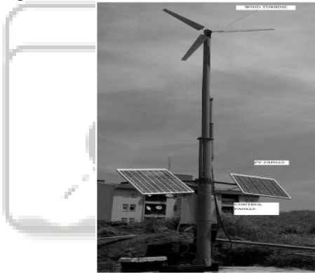
Fig. 4: A picture of the constructed hybrid system.
