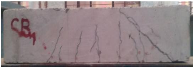
Fig. 1: showing the crack pattern of conventional beam
