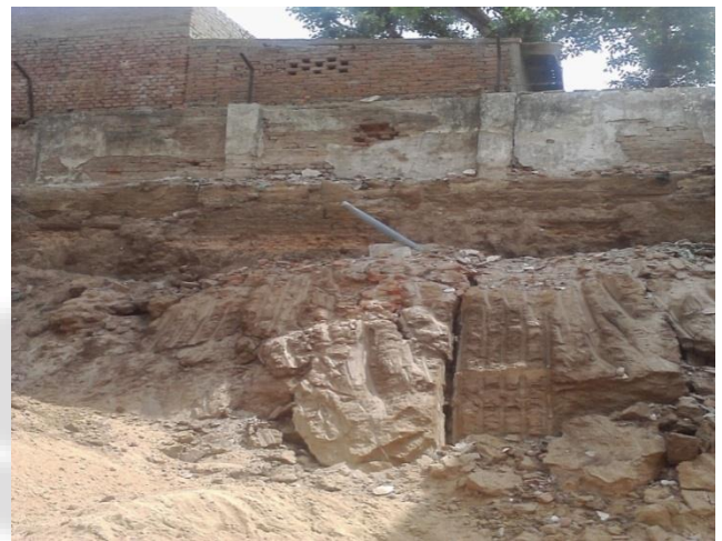
Figure. 3: Earth Collapse / Ground Failure
