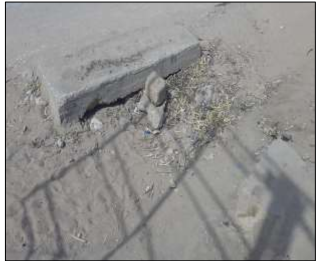
Fig. 7: The side drain is full of refuse dumps and dirty water.
