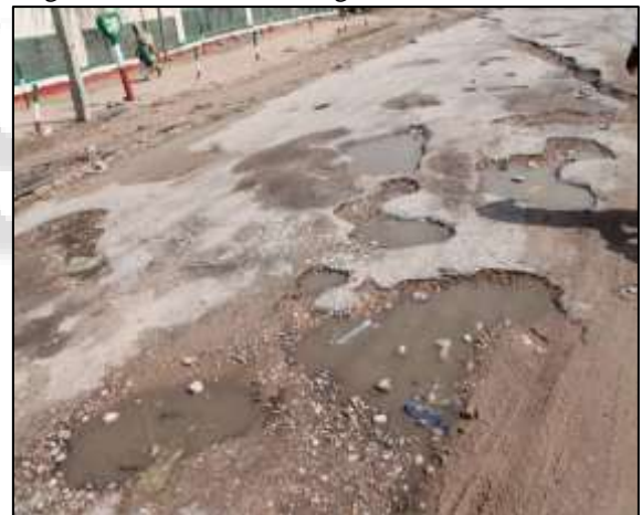
Fig. 8: Serve failure of road edge due to water ponding on surfaces.
