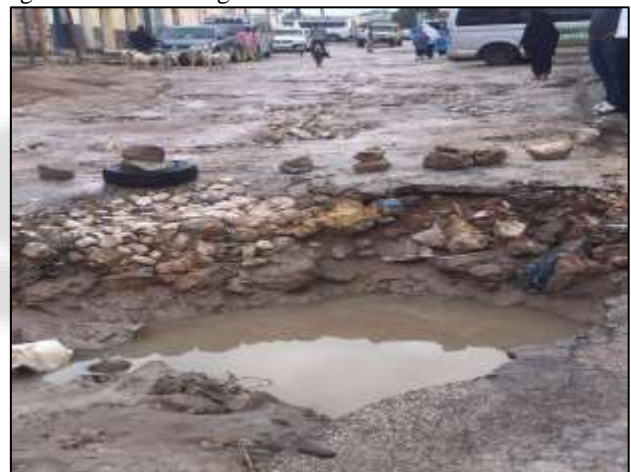
Fig. 5: Severe pavement distresses cracking, potholes, and failure edges.
