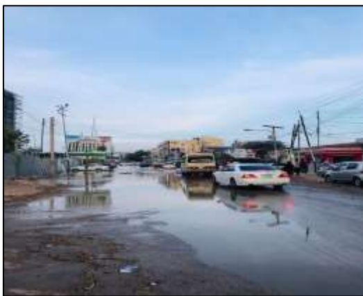
Fig. 4: The side drains and the culverts were blocked with sand accumulation garbage and roots.
