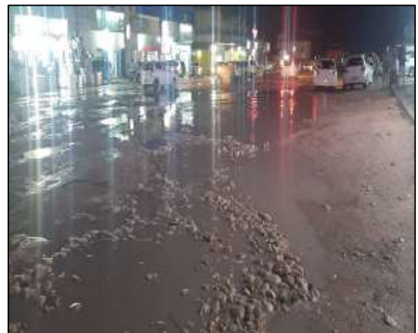
Fig. 9: Serve failure of edges and potholes.
